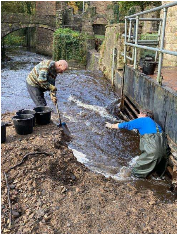
Inlet cleared, generation restarted, but still more 'beach' to clear
