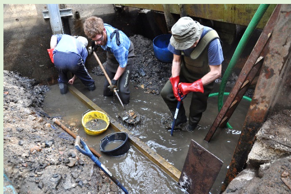
Volunteers digging out the silt to allow the bottom bearing to be replaced
