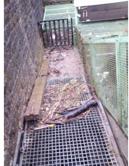
Debris on the fish pass steps
