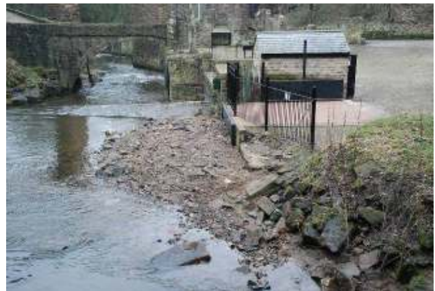
The 'Beach', rubble deposited by the rivers blocks the intake
