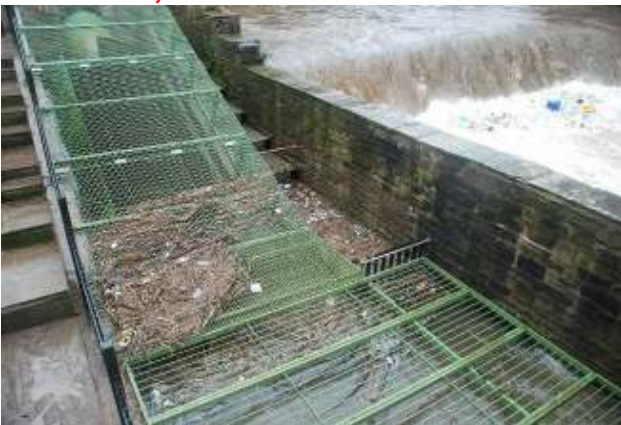
Debris on the cage while the river continues to rage
